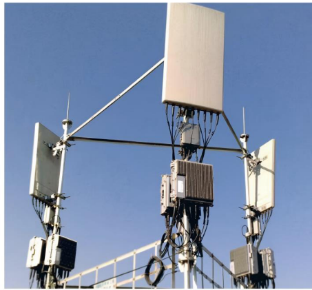
Communication base station
